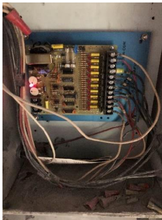
Fig. 2 – Example of aged baghouse control board
